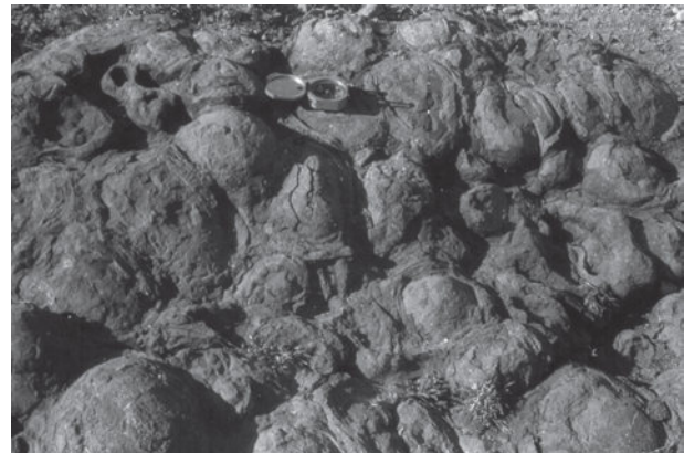
Fig.6.4 : Exfoliation (Flacking) and granular disintegration
